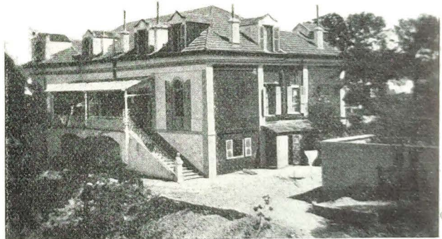
Hope House, prior to renovation. The roof is being raised and the upper rooms rebuilt.
