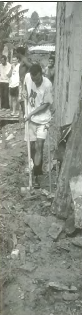
Jim Olinda. Above: Digging the trenches. Top right: Stuart Christine talking to one of the residents.
