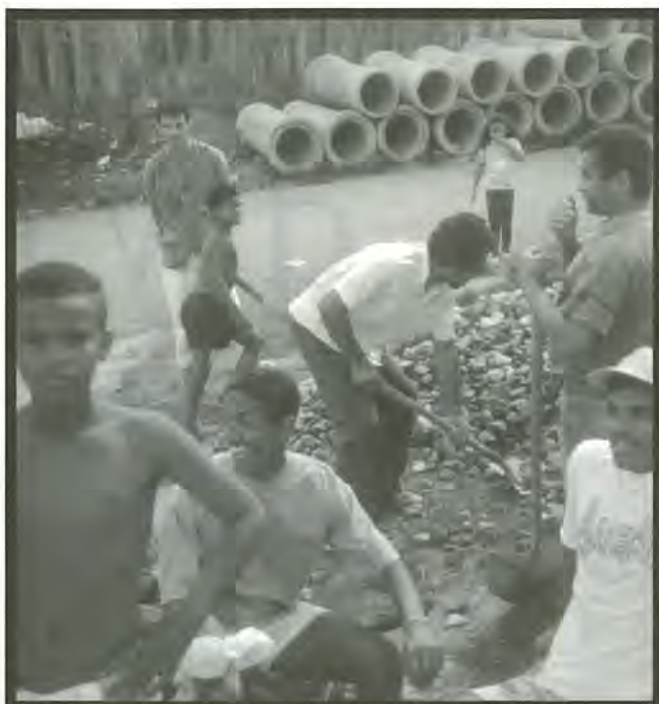
Getting ready to work on laying the sewer pipes in Jardim Olinda.
