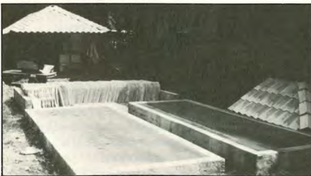
Above right: Cutting fibre for the tiles Above: Tiles at Butwal where the project was developed
