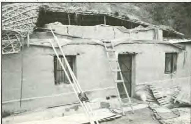
Cyclone damage at Chandraghona
