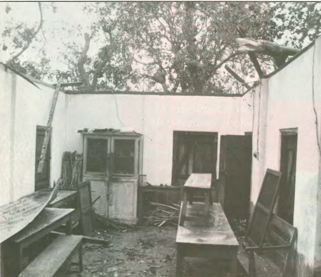
The damaged female nurses' dining room
