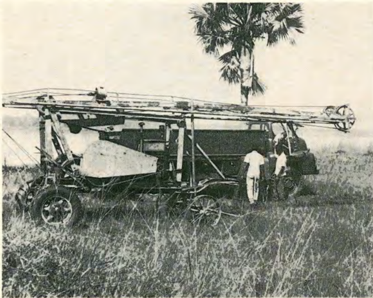
The somewhat ancient drilling rig which was used to sink the tube well. In the background the ex-army Bedford lorry which we use for all our heavy work. (Photo: P. Riches)
