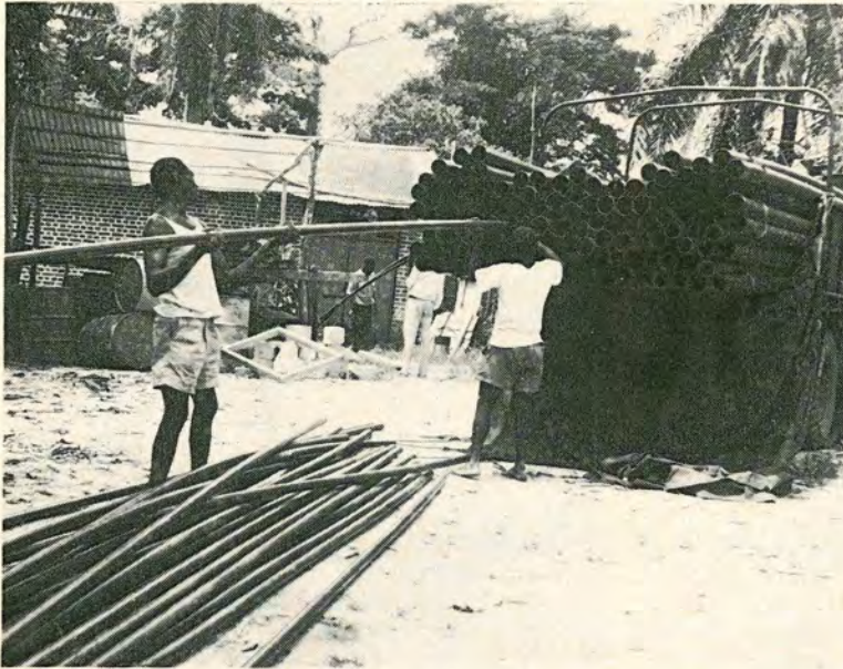
The first consignment of PVC water pipes for the mains distribution. There is a total of 850m of 4", 3", and 1½" pipes in this load.
