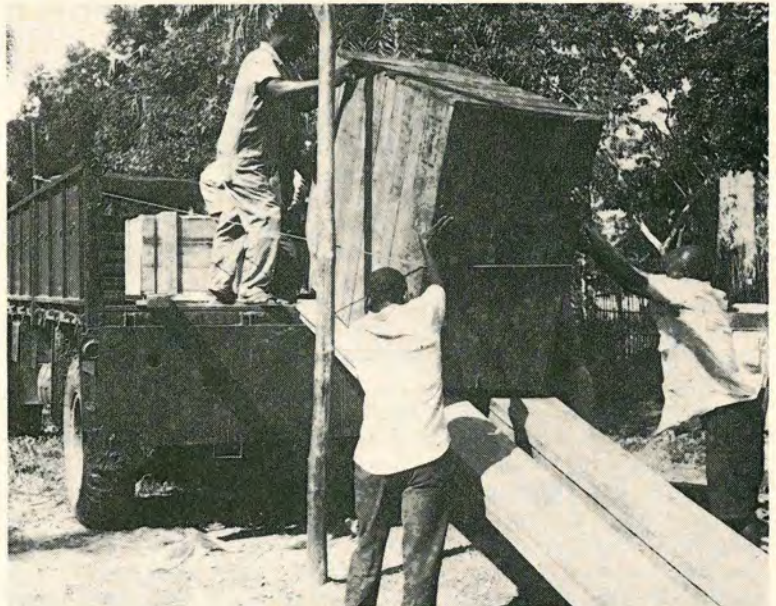
Unloading the new diesel generating set which now provides the power for the water pumps. (Photo: P. Riches)
